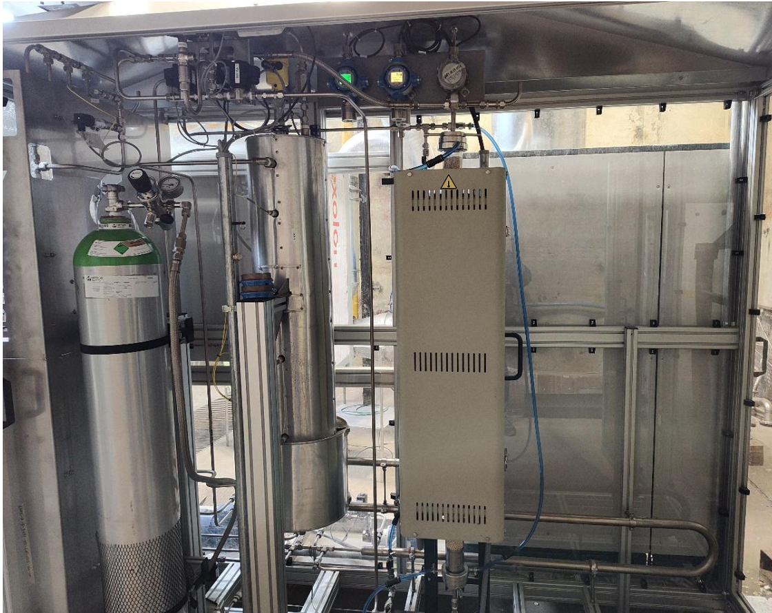
Overall view of the process area
